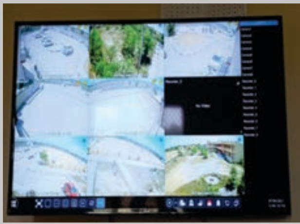
CCTV Setup in the College Premises
